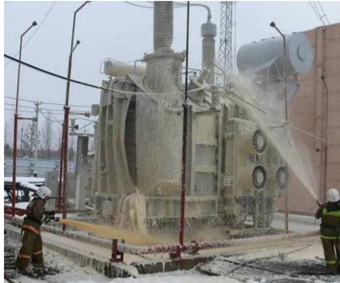
Figure 4 – Transformer in Western Siberia Substation after explosion
