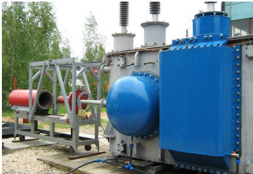
Figure 7 – Autotransformer with DPS before tests
